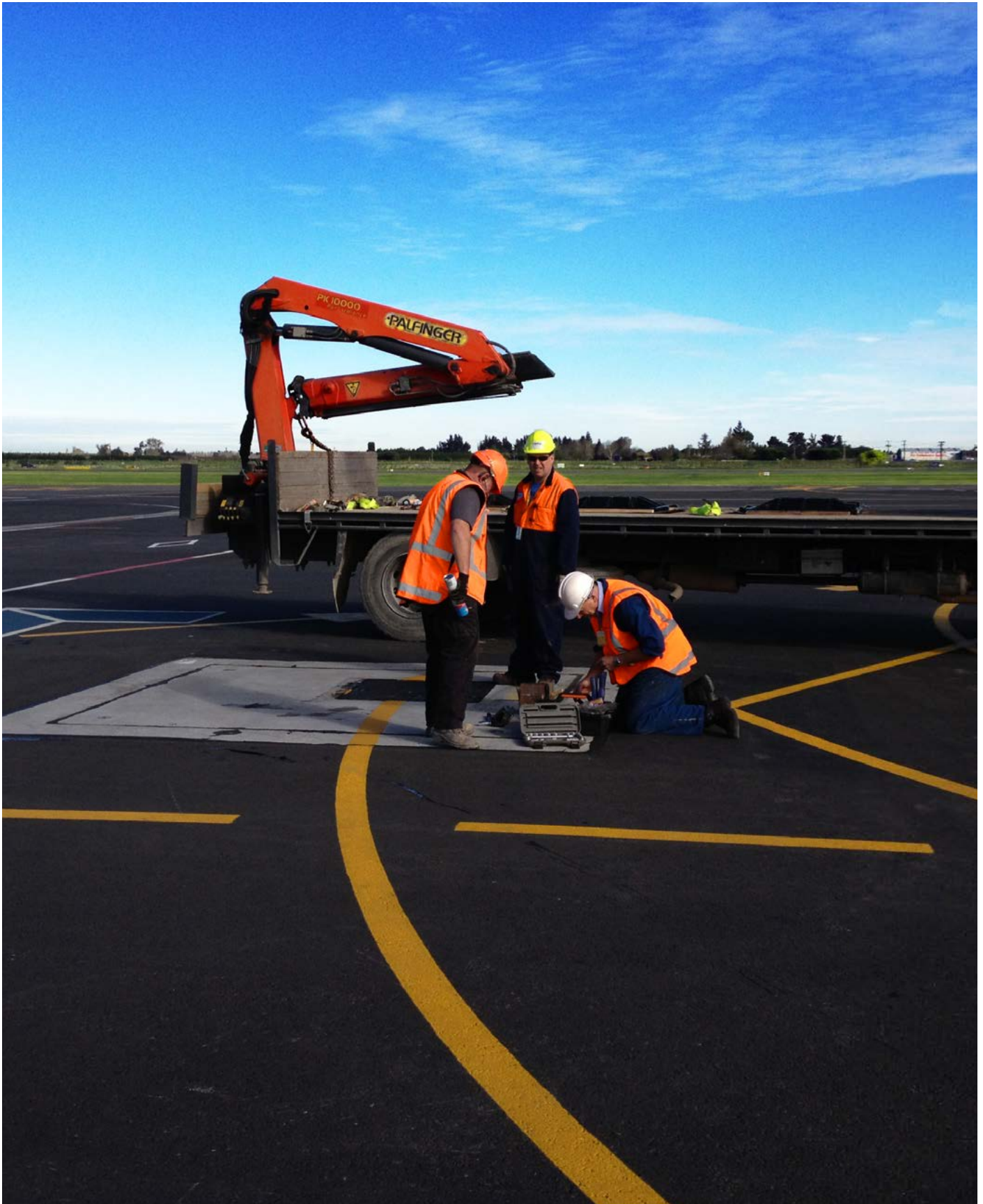
Christchurch International Airport, Christchurch, New Zealand - ERMATIC range
